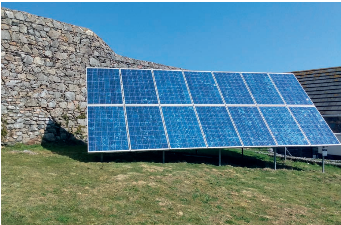
Power to the People winner. Live data screens installed for solar panels on Lihou.
