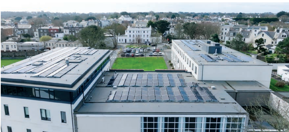
The installation of 292 photovoltaic (PV) panels on site at the Ladies College, make it the third largest PV scale on-Island and follows similar projects completed over the past three years at Guernsey Post, King George V Playing Fields and the Waste Transfer Station.
